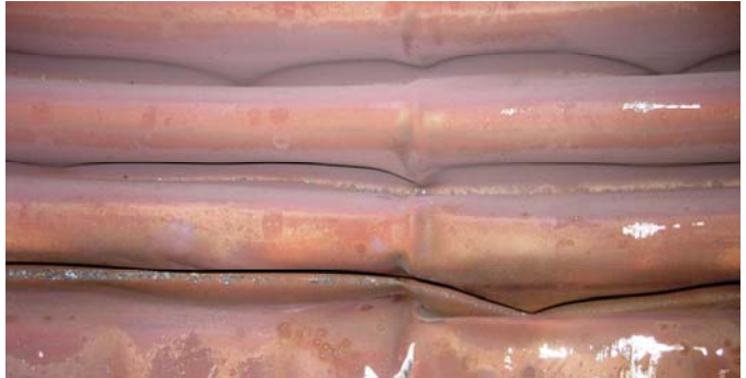
Imploded bellows inner ply with creases that will fail after a few cycles
